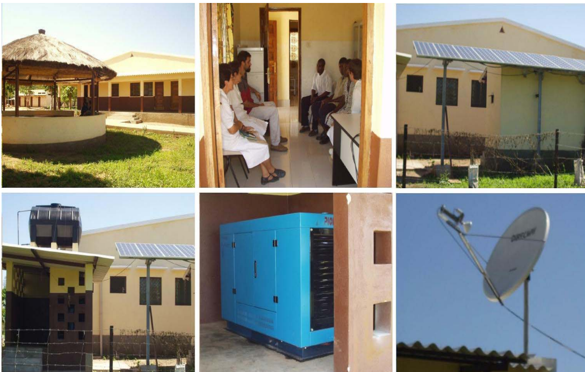
Figure 4B. Photos of Mangunde rural HIV clinic. Solar panels, a generator, water tanks, satellite dish have made it possible to establish the rural clinic in this remote area of Sofala Province.
