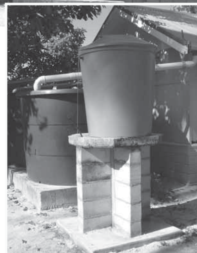
Support water tanks
